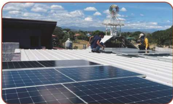
Complete Installation of Solar Panels and Submersible Pump System at Carangian, Tarlac
