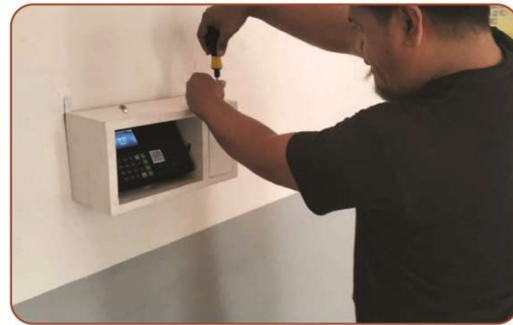
Deployment of ICT Devices
